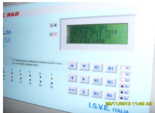
Figure 6. Control and heating unit of drying
