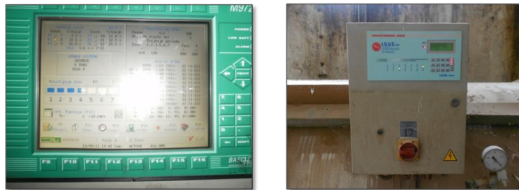
Figure 3. Automatic control system (convective drying and vacuum drying)
